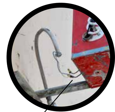
The exposed wiring outside of this sign cabinet is unsafe and non-compliant.
