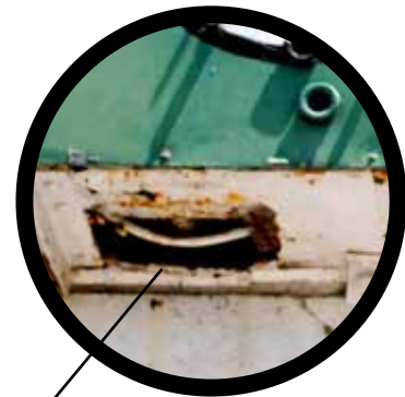
Exposed wire is unsafe. Unsealed access panel invites pigeons to nest. Bird guano will accelerate damage the metal cabinet.
