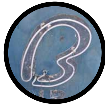
Exterior neon signs require repainting, approximately every six to ten years.
