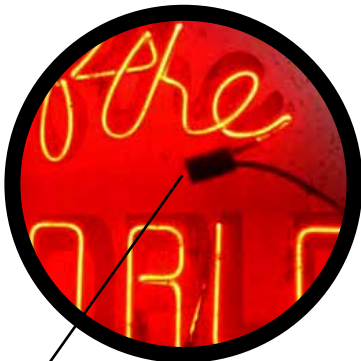
Rubber boots and wiring should never be outside of the metal cabinet as a repair shortcut on a vintage sign.
